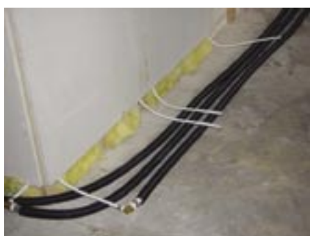
Connection of wall heating
